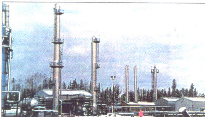
Poco Petroleum Ltd.'s O'Chiese gas plant in central Alberta added a 60-MMscfd enhanced absorption NGL-recovery unit.
